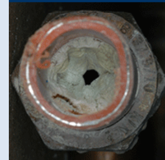
Corroded Kitec® Fitting
